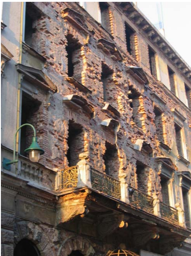
War damage in the centre of Sarajevo
