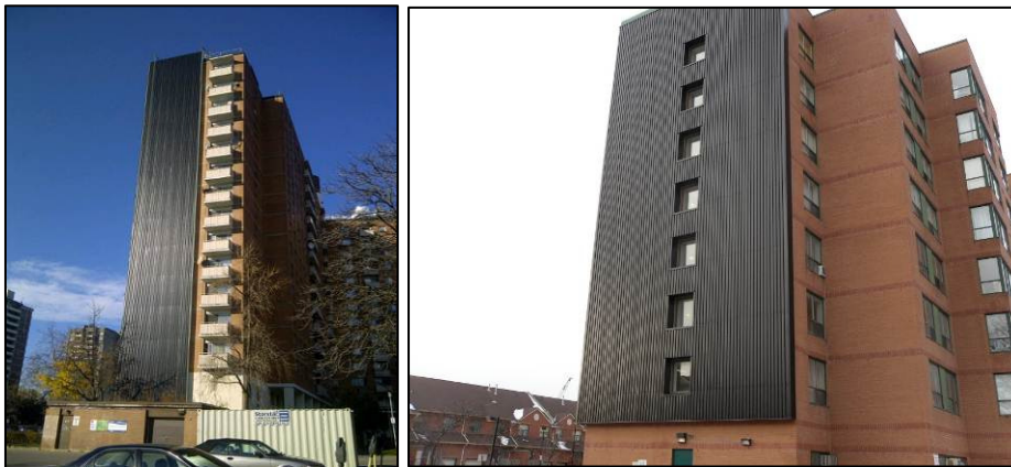
Figure 4 Solar Walls in two SHRRP Projects in Toronto. Source: City of Toronto, SHRRP Newsletter, 2011
